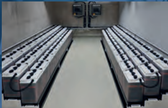
The battery system, configured for redundancy, ensures that the substation can continue to operate in the long term, even if there are disruptions to the external power supply
