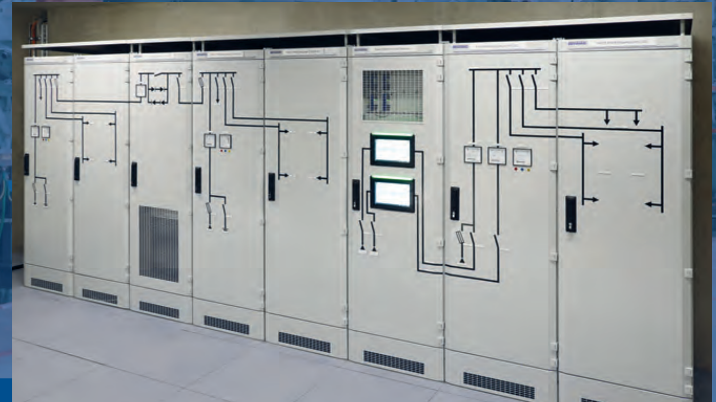
220 V and 60 V DC power supply system for the substation – with consumer distribution
